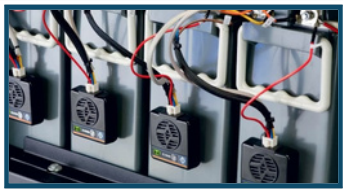
24X7 POWER BACKUP
